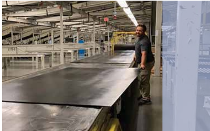
Featured here is our certified installation partner, SurfaceWRX, completing another successful TIVAR® DrySlide installation project.
